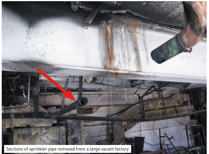
This vacant building was designed and constructed as an entertainment venue. Firefighters encountered heavy fire conditions due to abandonment of hundreds of rolls of carpet and rubber underlay inside the building. Note exposed and unprotected steel beams. Partial collapse of the building occurred
