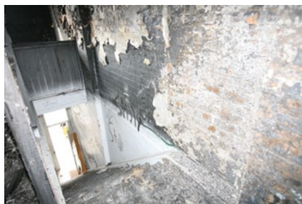
The access stairs to a vacant Newcastle shop. Firefighters were not expecting a ferocious flashover due to involvement of numerous polyurethane foam mattresses being used by vagrants
