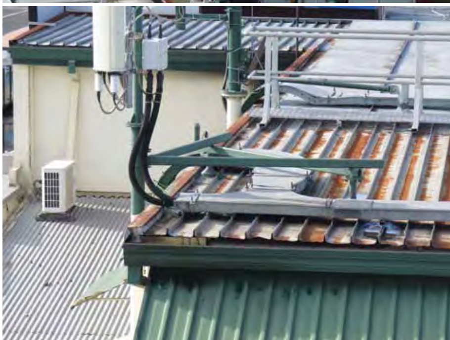
Power going to the roof mounted equipment is via DC supply and can only be isolated by the telecommunications carrier
