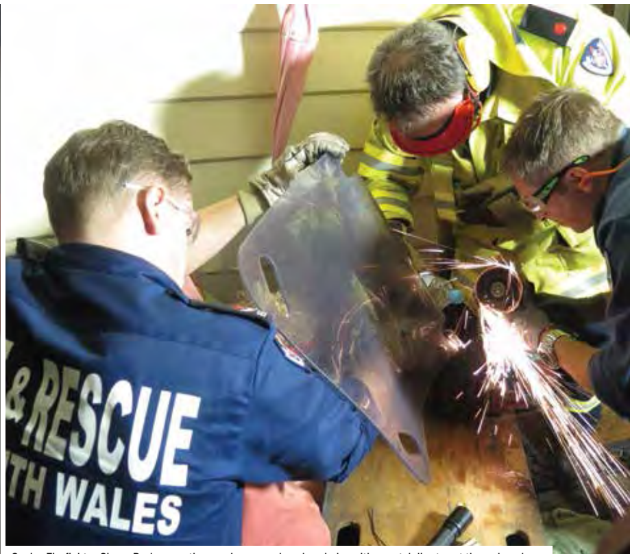
Senior Firefighter Shane Park, operating an air powered angle grinder with a metal disc to cut through and remove the section of the remaining bath tub from the drain plug. Cutting was delicate and precise at this time
