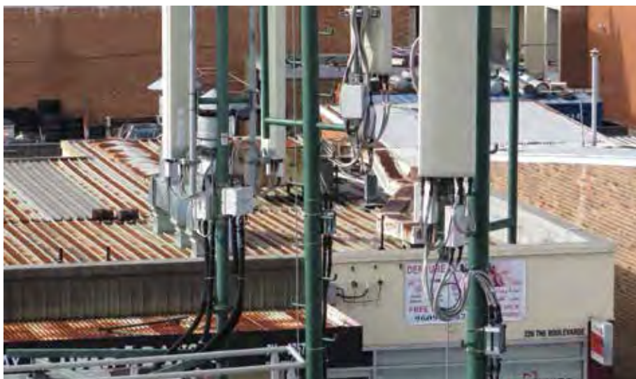
Receiving and transmission antennae located on the roof of the fire building, the most obvious sign a structure could be fitted with roof mounted mobile phone base station equipment
