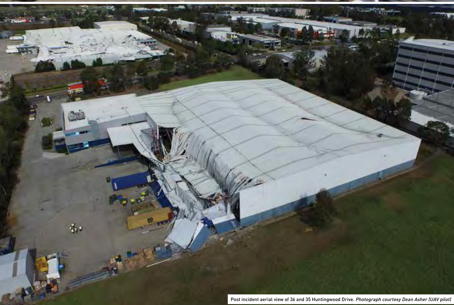
Many of the hazards at this incident can be seen in this picture, showing fallen concrete slabs, damaged electricity mains and broken sprinkler pipes
