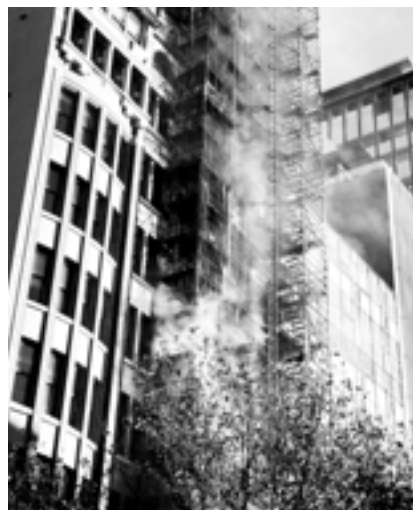
Scaffolding Fire at Macquarie Street, Sydney
