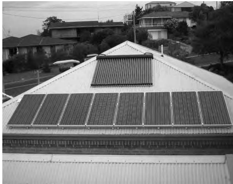
Solar hot water panels mounted on a fire station roof
