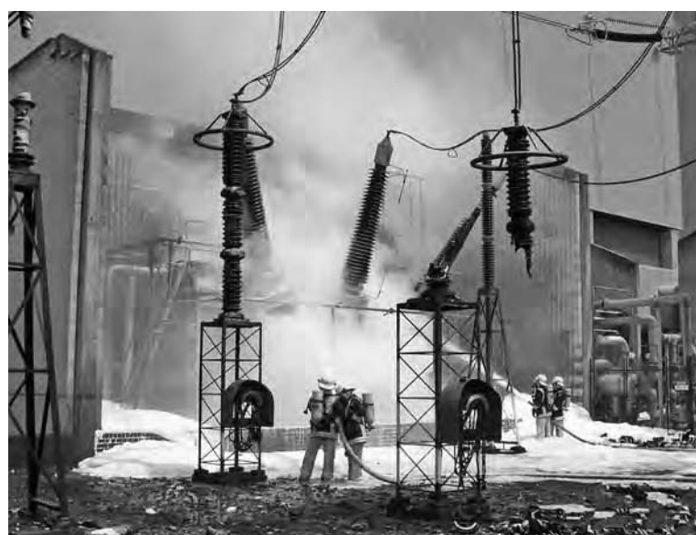
Fire officers using foam to extinguish a transformer fire at a power station
