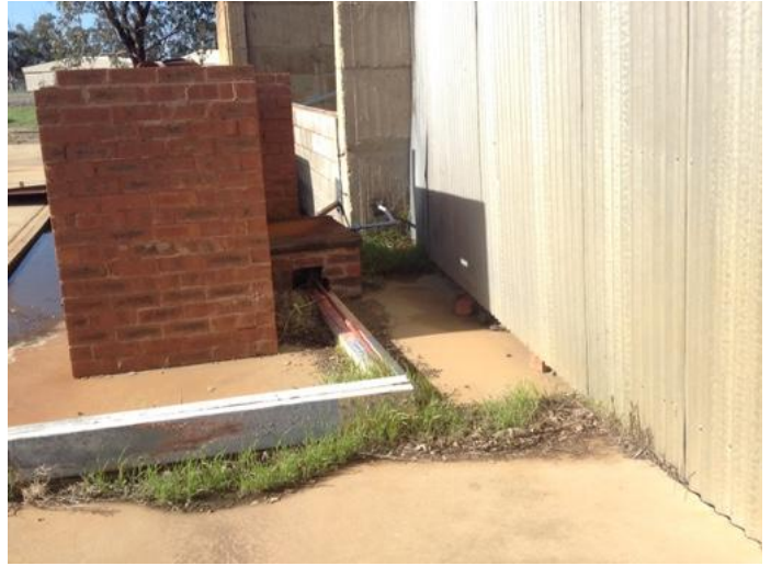
Appendix 2 – taken from where former AFFF use was, drain leading to pooling area in first photo
