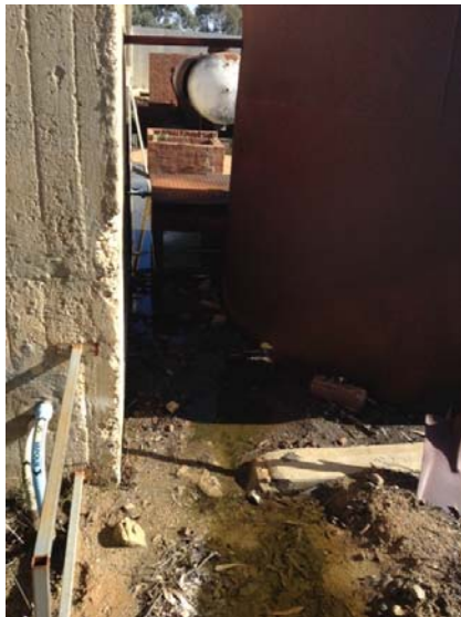
▲ Photograph 15: Water draining from bunded former foam training area to pooled water visible in Photograph 14.
