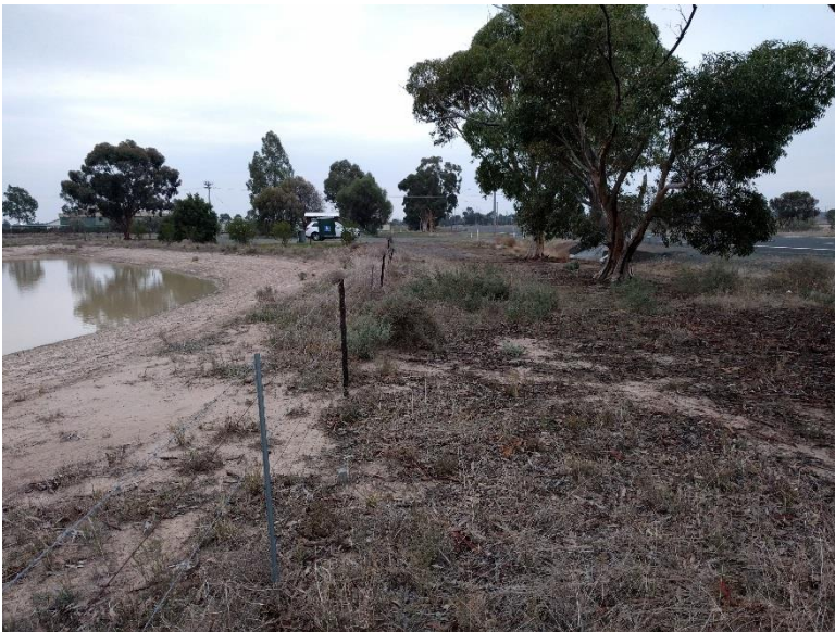
Photograph 10: Facing north, showing the new newly constructed dam and the culvert. No connection was observed between the drainage line and the dam.
