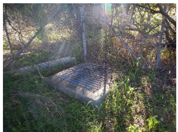
▲ Photograph 16: The north eastern stormwater pit in the corner of the site near the retention pond.
