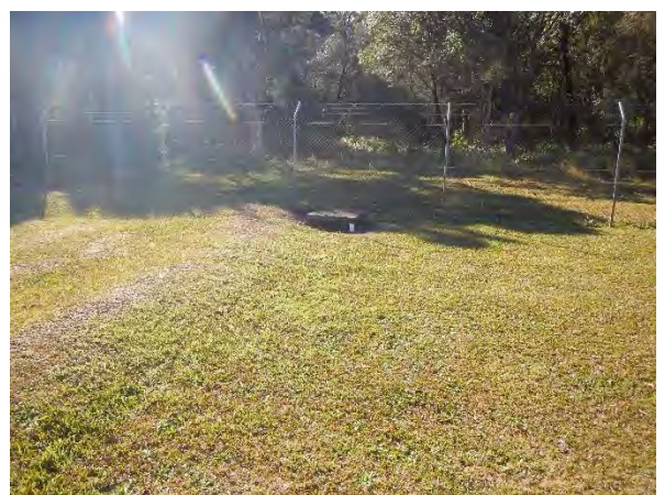
▲ Photograph 18: Large concrete drain collecting surface water on the eastern boundary of the site.
