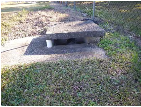
▲ Photograph 19: A close up of the stormwater drain in photograph 18 which shows the pipe direction to the north along the site boundary.
