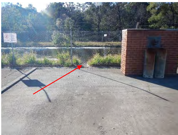
▲ Photograph 9: Facing east at the fire training props with the concrete drain which directs surface runoff into the retention pond.
